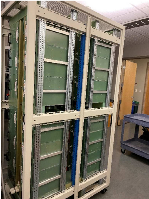
Fig.13. Full-scale power cabinet per arm.
