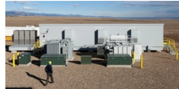
10 MW line capacity (upgrade up to 50 MW by 2015 with new 115 kV transmission line, NWTC on-site substation and 35.4 kV collector system)
